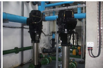
Final water PS at Desalination Plant
