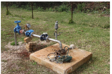
Kurland Borehole No1 (Yield 3 l/s)
