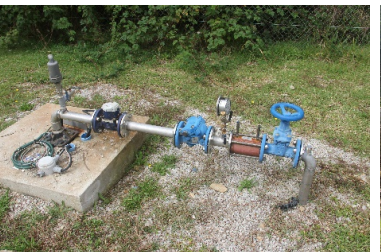
Kurland Borehole No2 (Yield 4 l/s)
