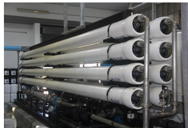
Three banks of RO Membranes
