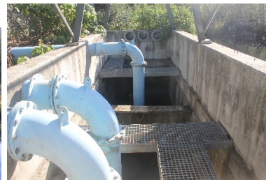
Keurbooms raw water PS inlet pipework
