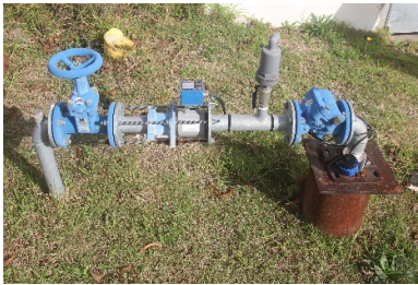
WTW Borehole No.3 at WTW
