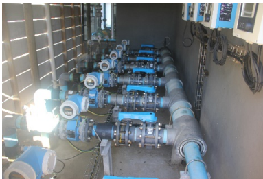
Seven inlets for Desalination Plant
